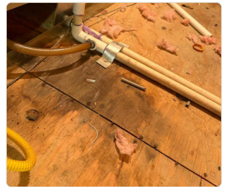
Plate 37. Platform deck: loose insulation fragments, pipe offcuts and metal debris left in place.
