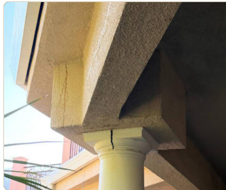
Plate 51. Beam over a column; a crack passes through the capital block at the bearing point.
