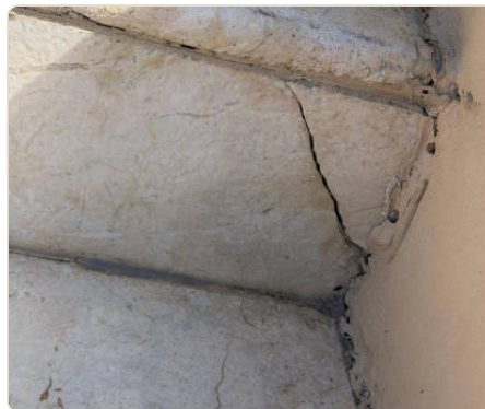
Plate 03. Stone-clad step, tread cracked through and separating at the wall junction.
