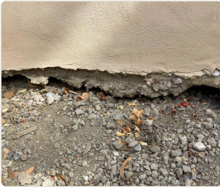
Plate 12. Base coat overhanging open voids; soil removed from beneath the wall line.
