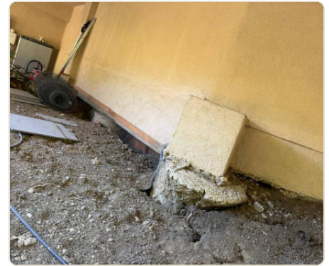
Plate 52. Interior space with a bare soil floor; wall base above a broken, spalled foundation corner.
