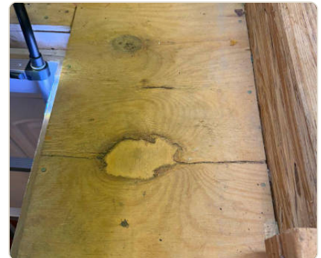
Plate 44. Plywood deck with a defined stained patch and a split running from it along the grain.
