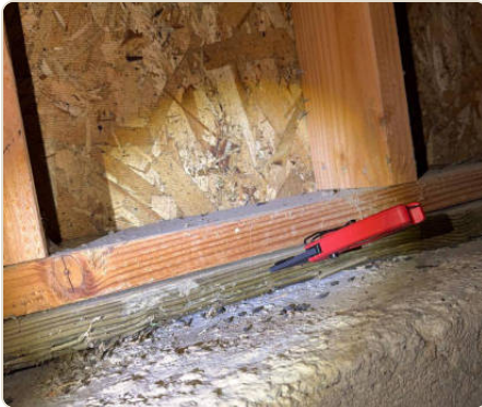
Plate 27. Mudsill on the foundation top with a heavy white crystalline bloom on the concrete below it.
