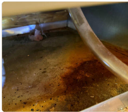
Plate 39. Close view inside the pan: heavy orange rust, dark deposits, cobweb and debris.
