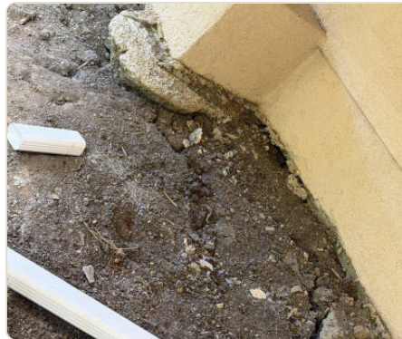
Plate 20. Base coat broken and crumbling at a corner; loose downspout section on the soil.
