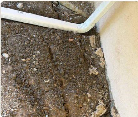
Plate 17. Downspout turning to discharge at the wall base; soil below scoured into a trench.
