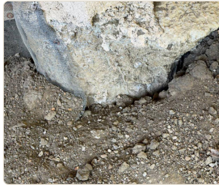
Plate 18. Corner with lath reinforcement exposed and hanging free, concrete edge broken away.
