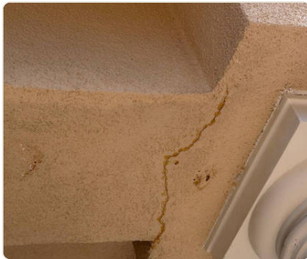
Plate 10. Crack down a beam face beside a column, with amber-brown staining along its full length.
