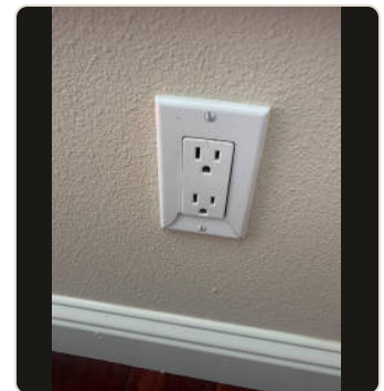
Plate 32. Cover plate cracked through.
