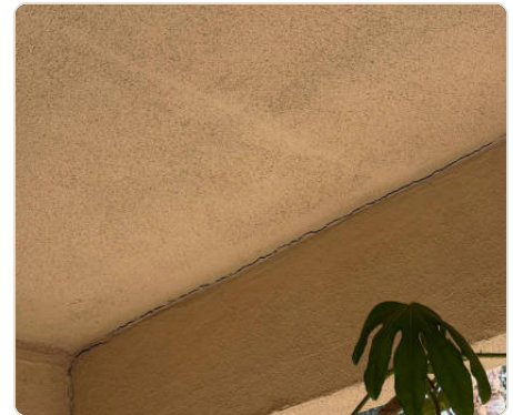
Plate 11. Long open crack along a soffit-to-beam junction, running the length of the frame.
