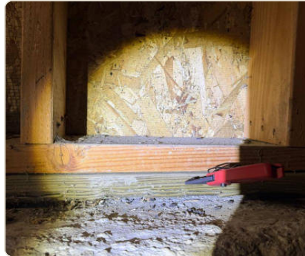
Plate 28. The same deposit in an adjacent framing bay, extending onto the soil.
