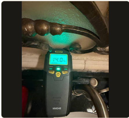
Plate 23 — 14.0%. MID lamp lit, at a plumbing fitting.
