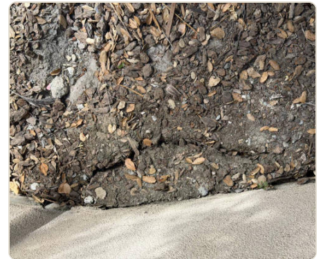
Plate 21. Soil and organic debris banked in direct contact with the wall base.
