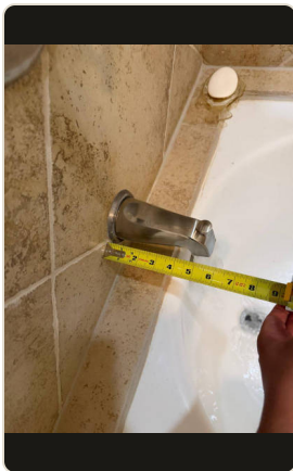
Plate 34. Tub deck at the spout. Grout and tile substantially discolored throughout this enclosure.
