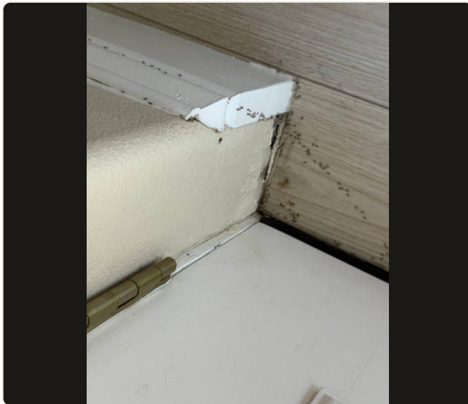
Plate 49 • Exterior door frame. A substantial number of small insects on and around the painted frame and jamb, concentrated at an open joint in the trim. Dirt streaking runs below the joint. Photographed as found; no specimen was collected.
